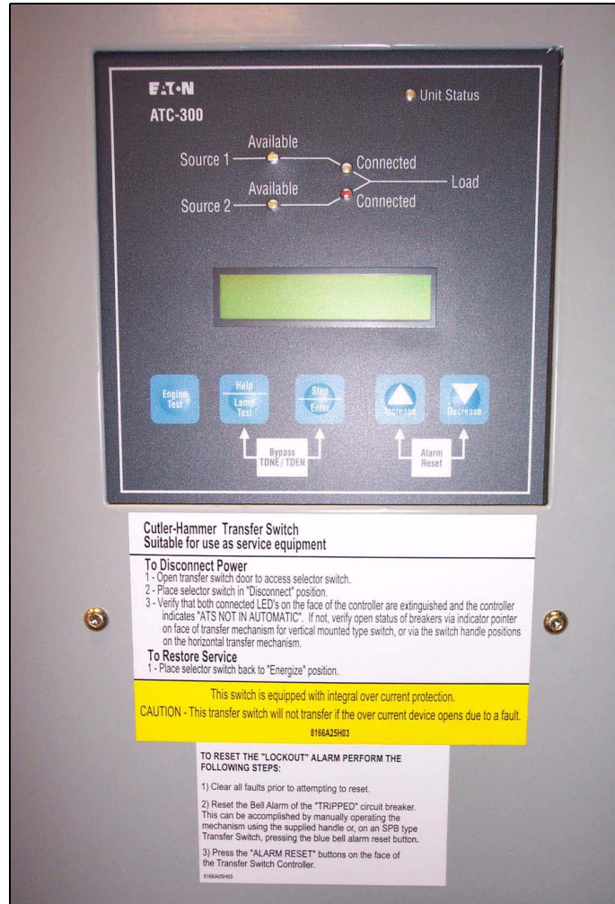
Figure 15. ATC-300 Logic Control Panel.
