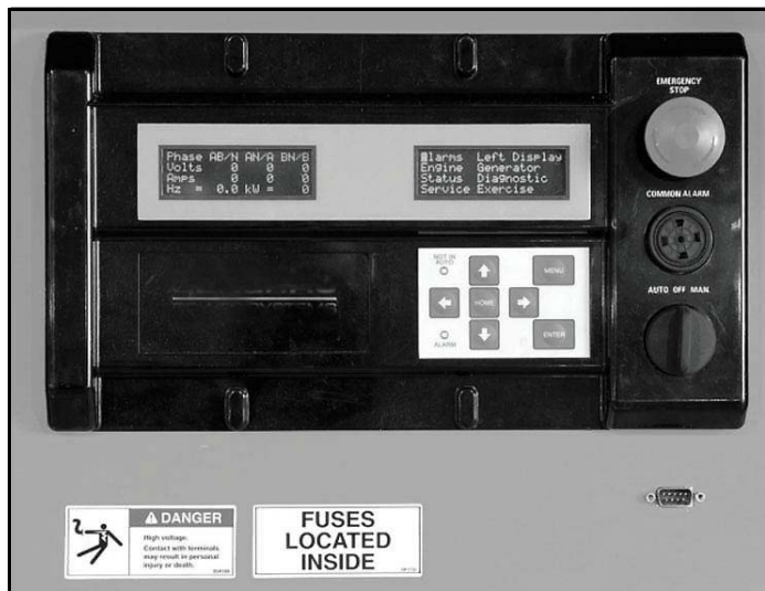
Figure 3-2. H-100 Control Panel Interface
